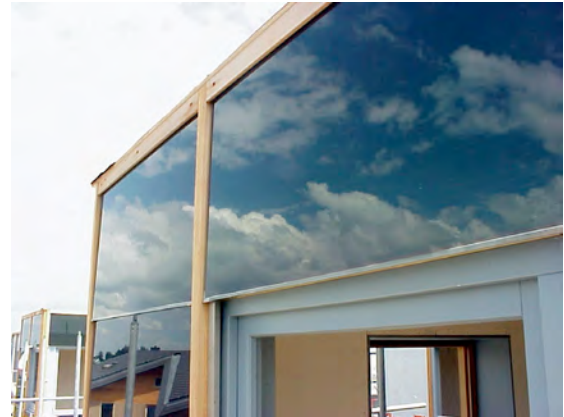
PV rain screen cladding on a Solarium
